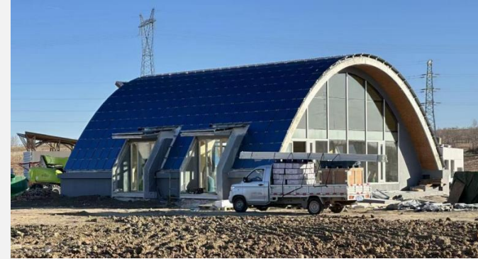
Solar Ark 5.0 Project
